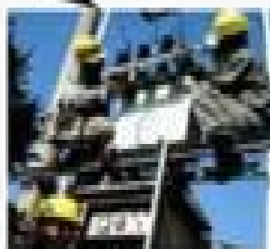
Monitoring the power supply transformer
